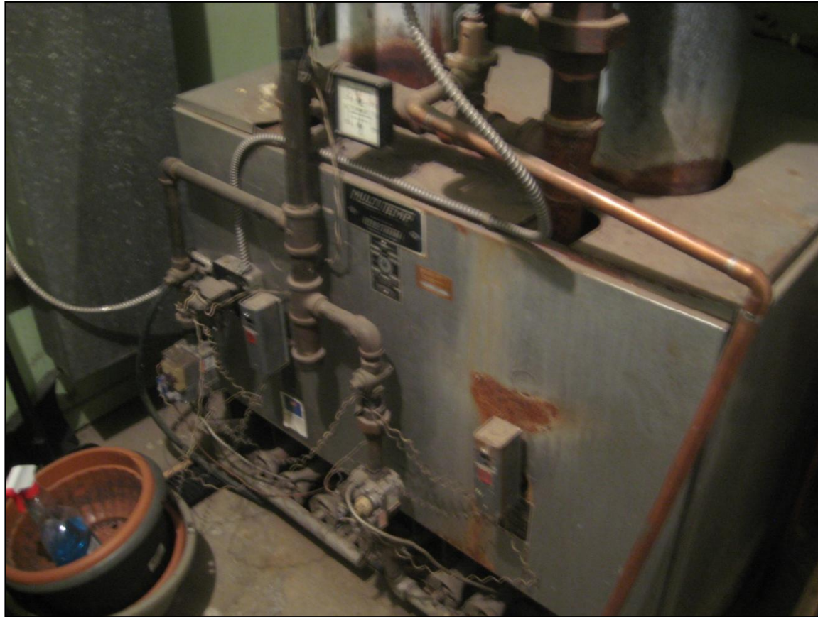
Condo Conversion – “New Boiler”
